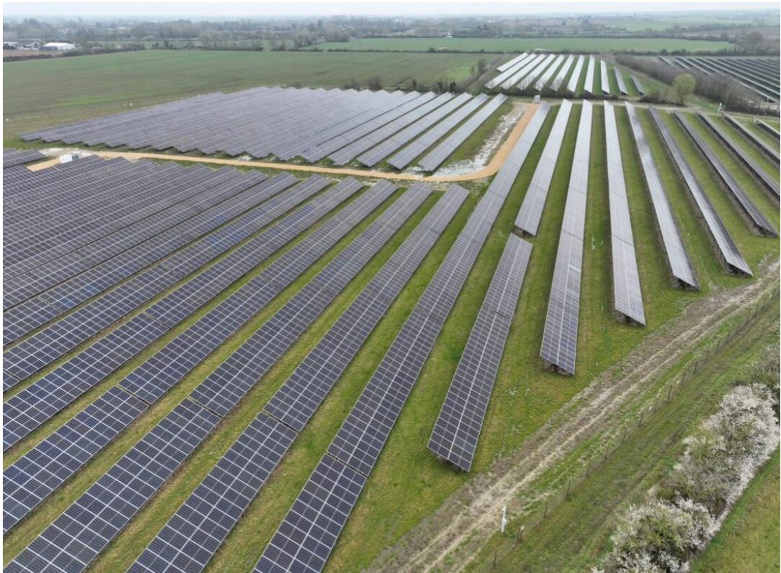
FIGURE 9.1 – EXAMPLE OF SOLAR ARRAYS
